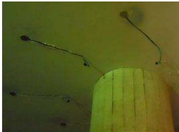
Furrows of the electrician after the paiter did his job
